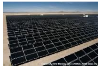
430 kW PV array Scaled to 19.3 MW
