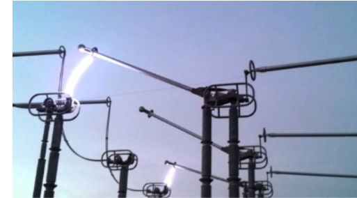
Opening HV Air-break disconnect under load (Not supposed to happen, but still cool!)
