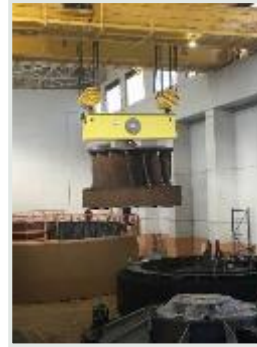
Denison Dam Turbine
