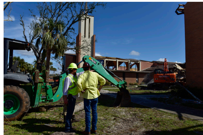
Construction Workers Survey the Base Chapel Before Demolition U.S Air Force Photo by Staff SGT Alexandre Montes
