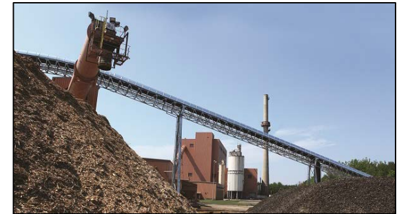
28 MW Biomass Plant Fort Drum, NY, Feb 2014
