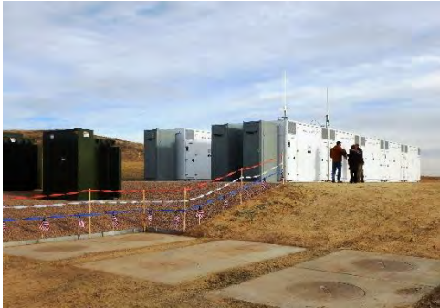
Battery Energy Storage System Fort Carson, CO
