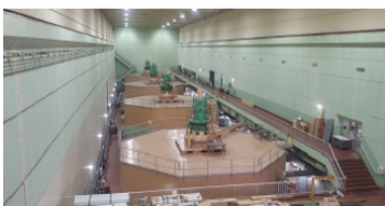
RS Kerr Powerhouse
