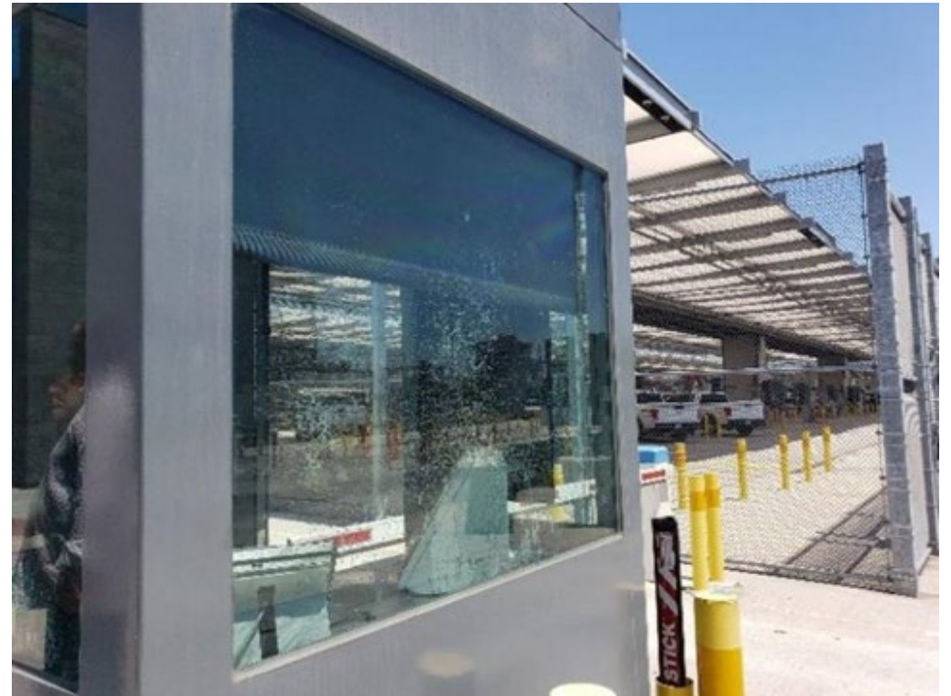
Shattered bullet-resistant glazing at Calexico Land Port of Entry.
