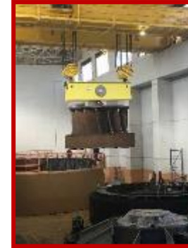
Denison Dam Turbine
